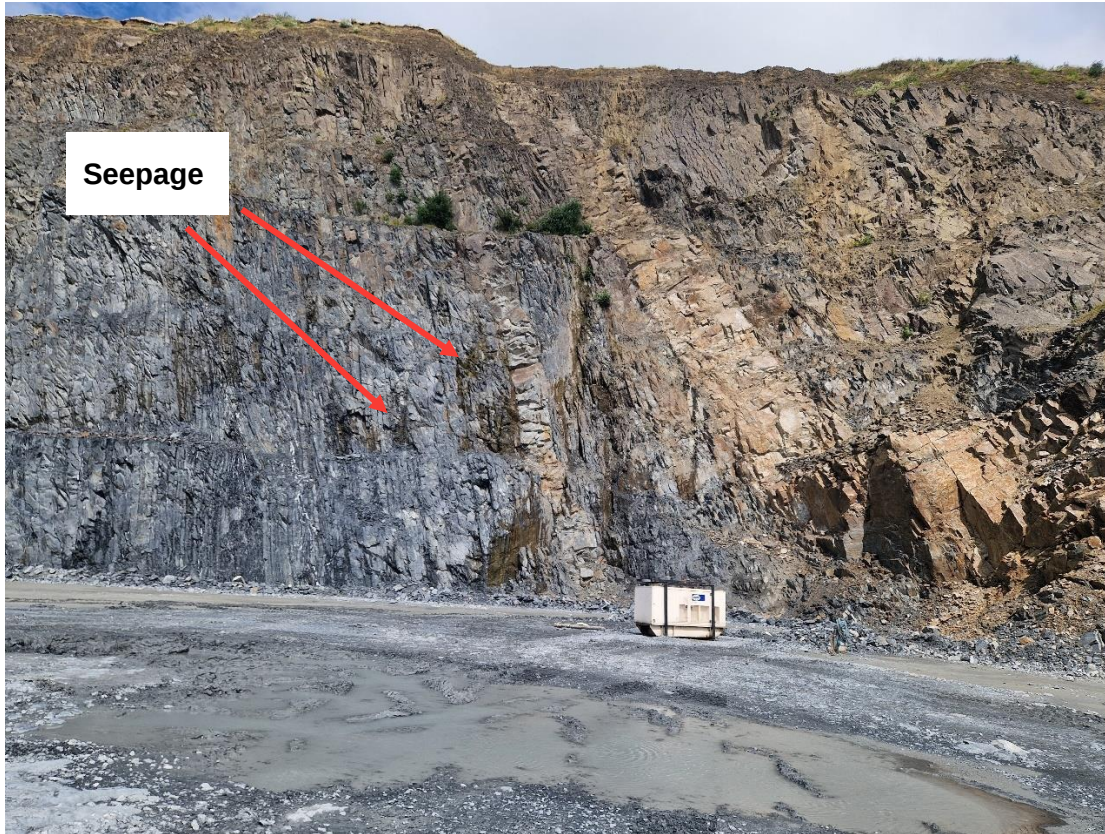
Figure 6-2 - Eastern Wall Seepages
