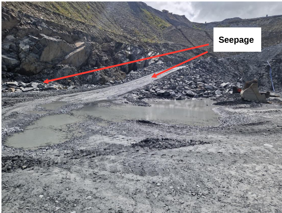
Figure 6-4 - Southern Wall and Ramp Seepages
